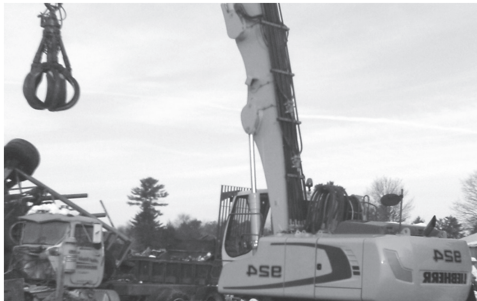
Earth Waste Systems recently added this Liebherr 924 Crane to move material at their Castleton location.
