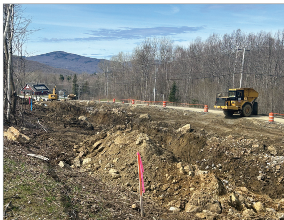
The west side of Killington Road is dug out, blasting to come.
