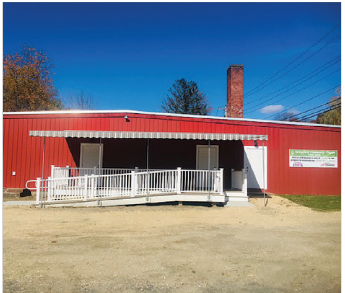
Courtesy of Springfield Community Players The Springfield Community Players’ South Street studio roof requires funding to replace its existing roof.
