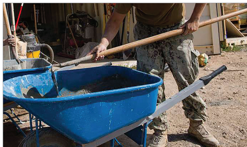
Submitted Concrete was mixed and carried in a wheelbarrow to build the lodge foundation.
