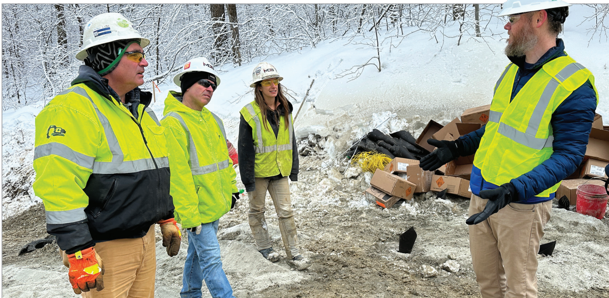
By Polly Mikkula Top left: Guy Keefe points to blasting holes before the explosion Wednesday, Jan. 31. Top right: Killington Town Manager Michael Ramsey examines the blasting site after the explosion. Below: (l-r) Charlie Wadleigh, Keefe, Elissa Spagnola and Ramsey.
